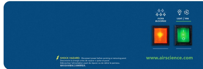
Basic Control Panel
